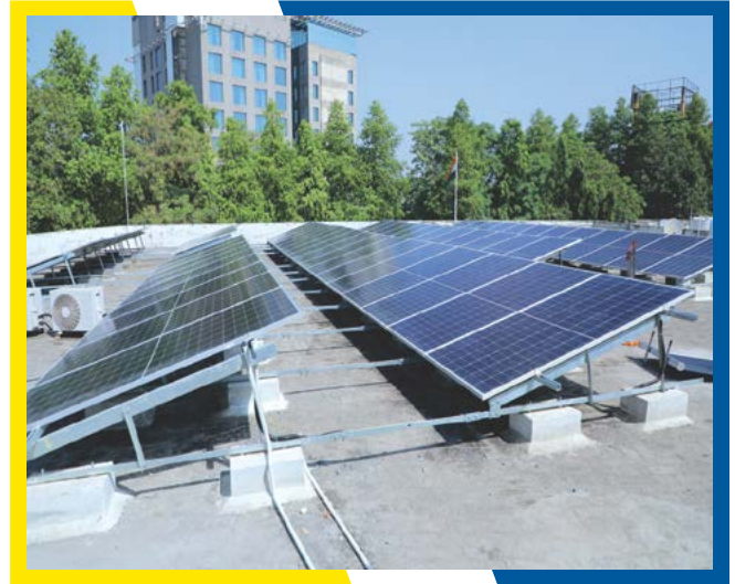
35 kWp capacity Solar Plant installed at Office of Commissioner of Police, Faridabad
